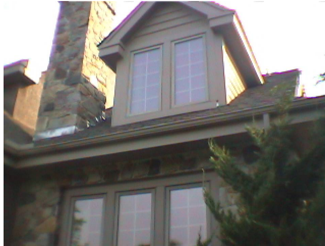
Rot on the left rear and loose trim on front
